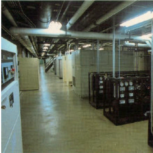
Figure 22. Systems are on UPS with battery and three diesel generators.
