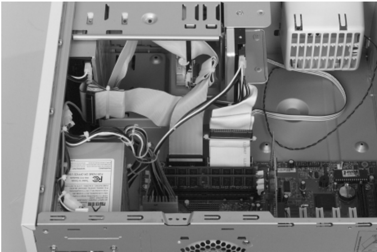
Photo 44. Cables Rerouted Using Tiewraps
